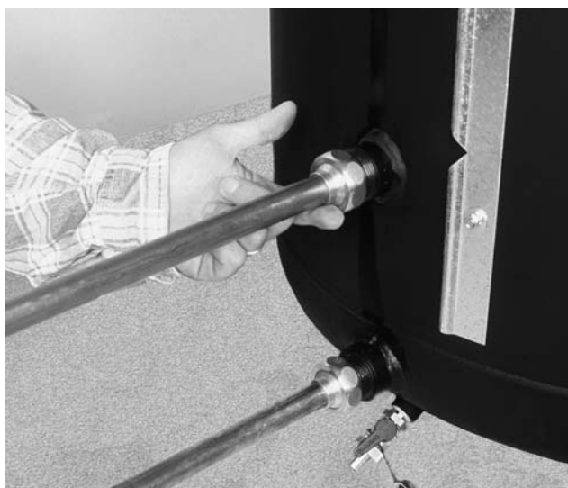
Figure 17 Check all connections and flanges for leaks after applying the test pressure.
